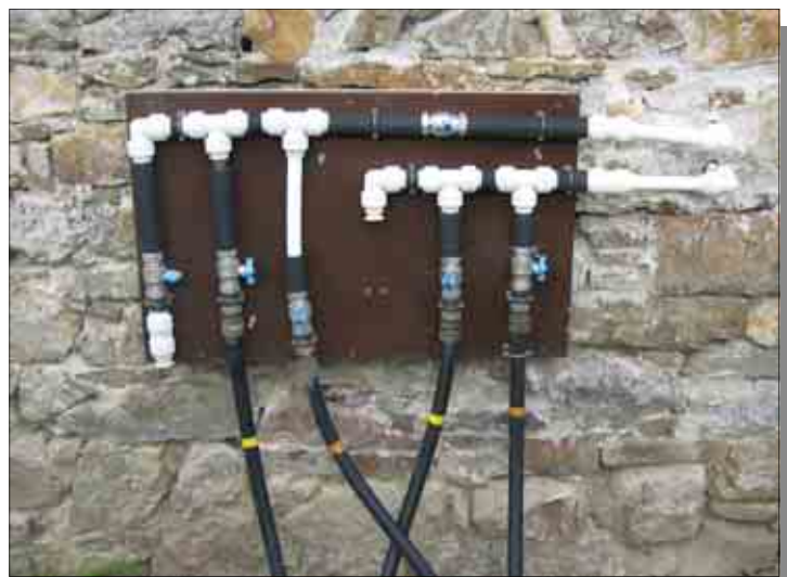
The Heat Pump Manifold at Old St. Lawrence
